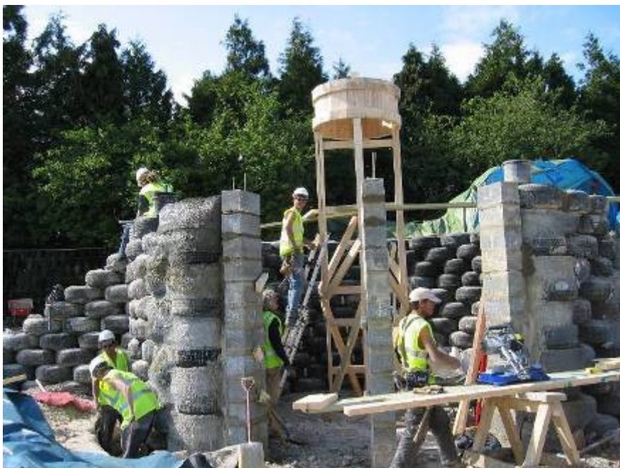
Figure 6: Construction of the hut module, Brighton Earthship, 2004 (Howarth, 2004) (The completed hut is shown on the picture on the front cover).
