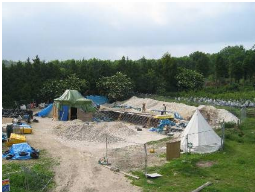
Figure 4: Construction of the nest module thermally massive rear wall, Brighton Earthship (Hodge, undated).
